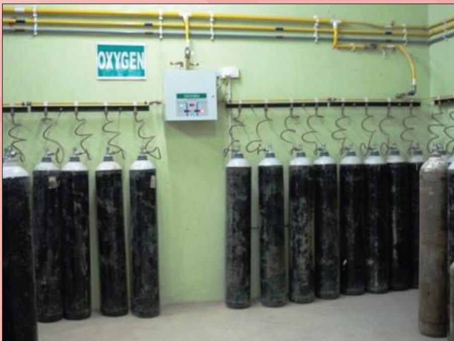
Oxygen manifold (Source: http://www.ijaweb.org/article.asp?issn=0019-5049;year=2013;volume=57;issue=5;spage=489;epage=499;aulast=Das )
