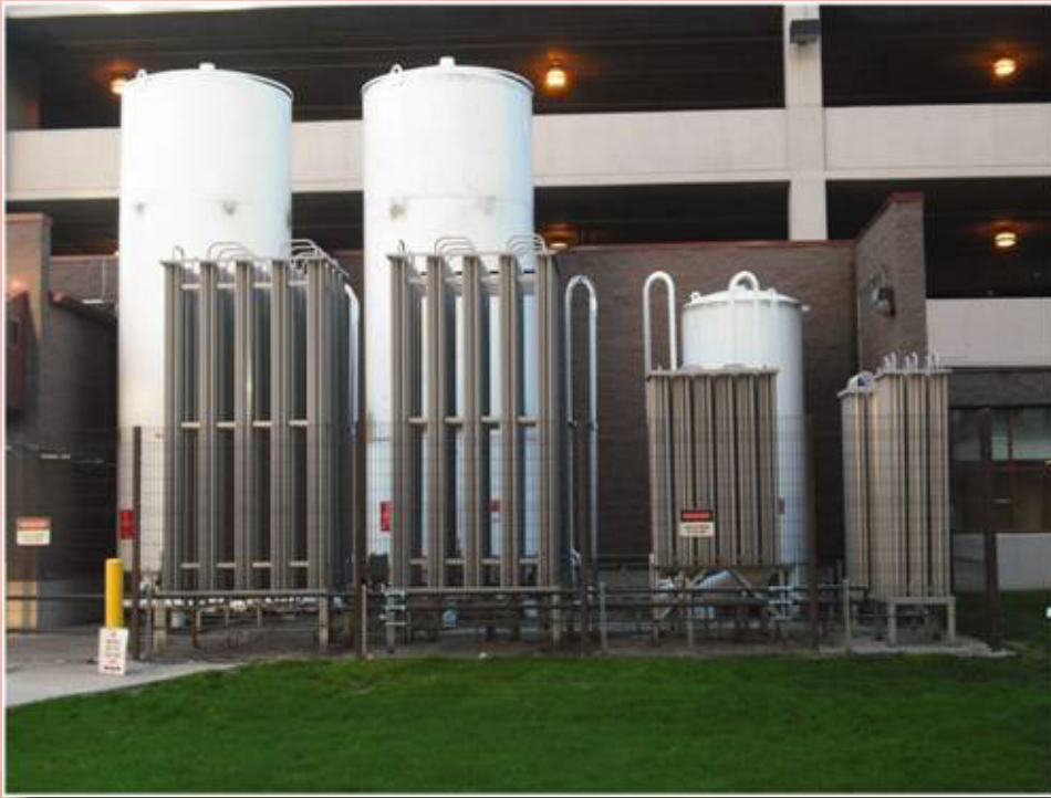
Liquid oxygen installation (Source: http://rc.rcjournal.com/content/58/1/173 )
